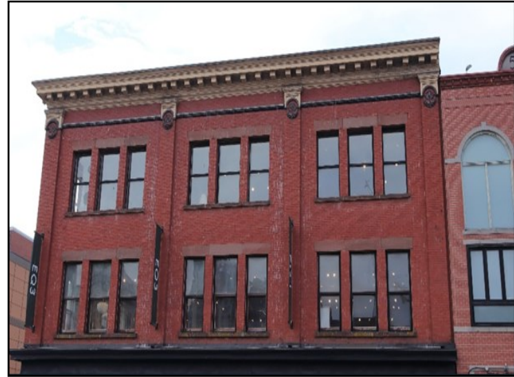
Figure 11: An example of distinct and eye-catching roofline with preservation of the original cornices defining the upper edge of the building's façade.
